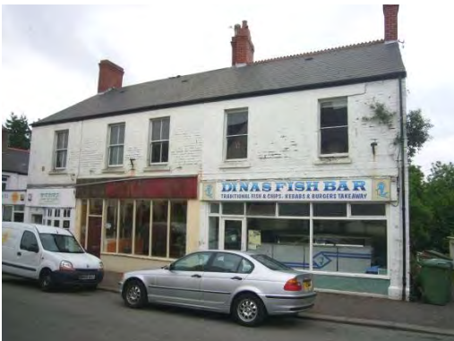
These buildings are in need of routine maintenance.
