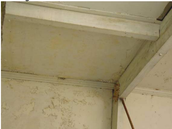
Plate 17: Gaps between plaster roof and slates at south of building 4
