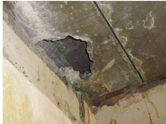
Plate 20: Holes in concrete ceiling of building 5
