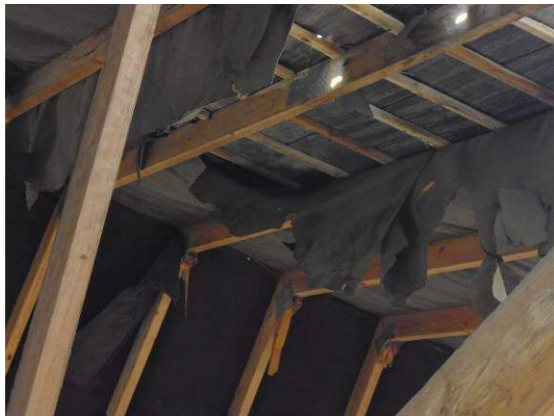
Plate 5: Loose lining within building 1
