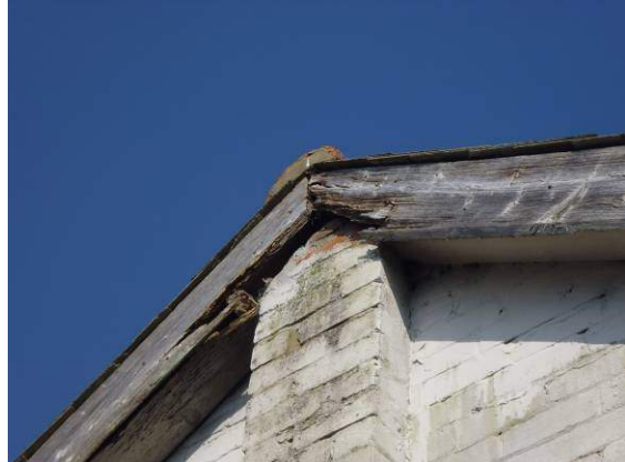
Plate 14: Eroded bargeboards at southern elevation
