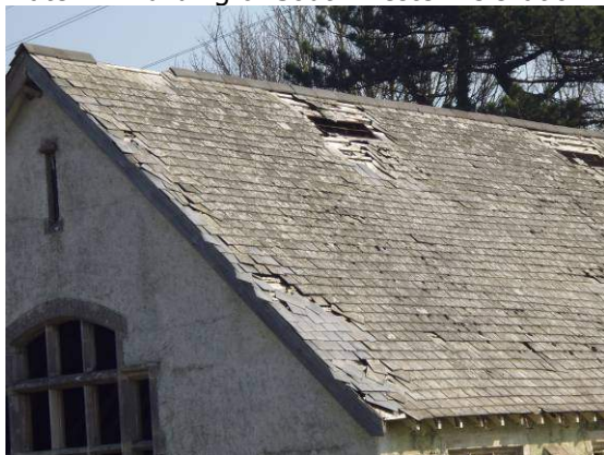
Plate 23: Building 6: Slipped tiles and gaps in roof
