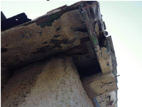
Plate 11: Gaps into soffits of building 3
