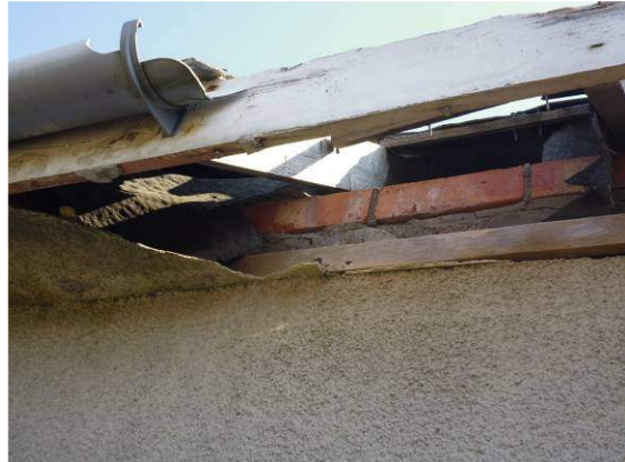
Plate 2: Eroded soffit of building 1
