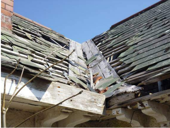
Plate 7: Numerous missing tiles and exposed cavities behind fascias of building 2
